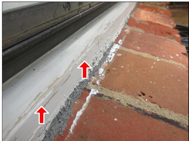
2.0 Item 8(Picture) Flaking Paint
