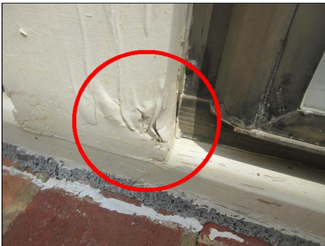
2.0 Item 7(Picture) Damaged
