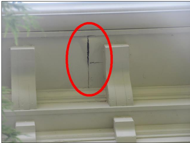
2.0 Item 2(Picture) Damaged
