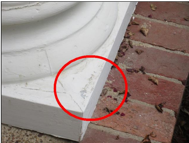
2.0 Item 5(Picture) Flaking Paint
