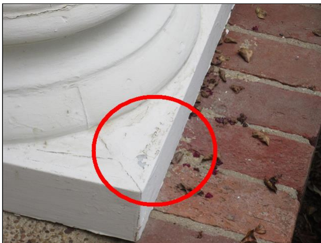
2.0 Item 5(Picture) Flaking Paint
