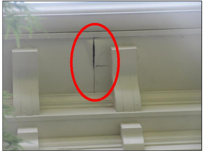
2.0 Item 2(Picture) Damaged
