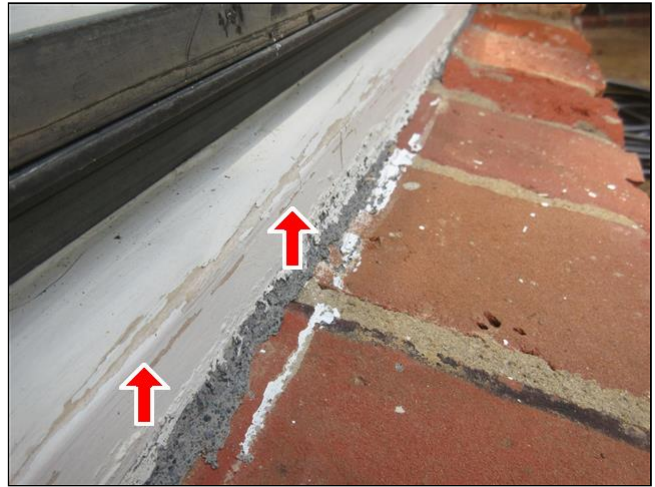
2.0 Item 8(Picture) Flaking Paint
