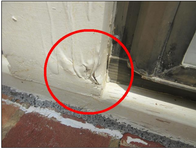
2.0 Item 7(Picture) Damaged
